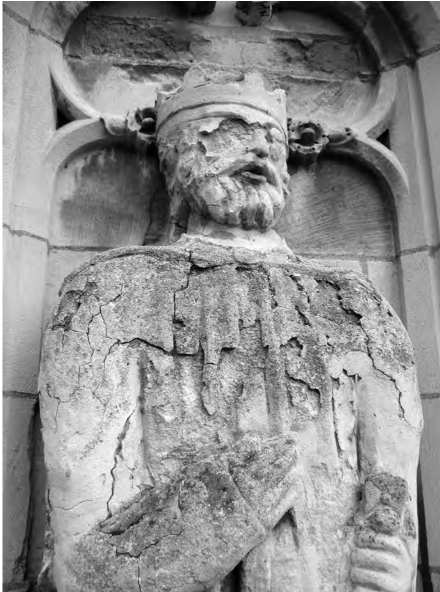
Figure 9.4 Beer limestone statue of Edward the Confessor, early nineteenth century, Exeter Cathedral West Front. There is deep decay under the hard impervious cement repairs, which are cracking and falling away.
