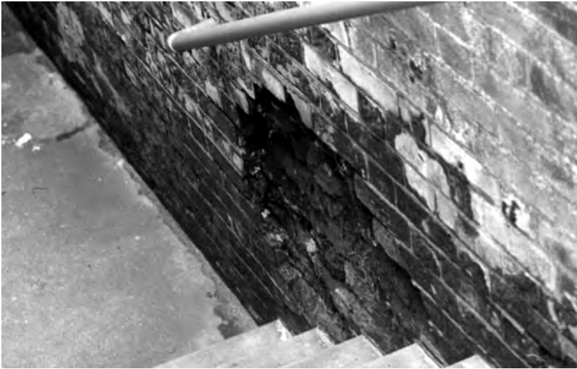
Plate 9.4 Frost damage is usually worst in walls that are permanently soaked.
