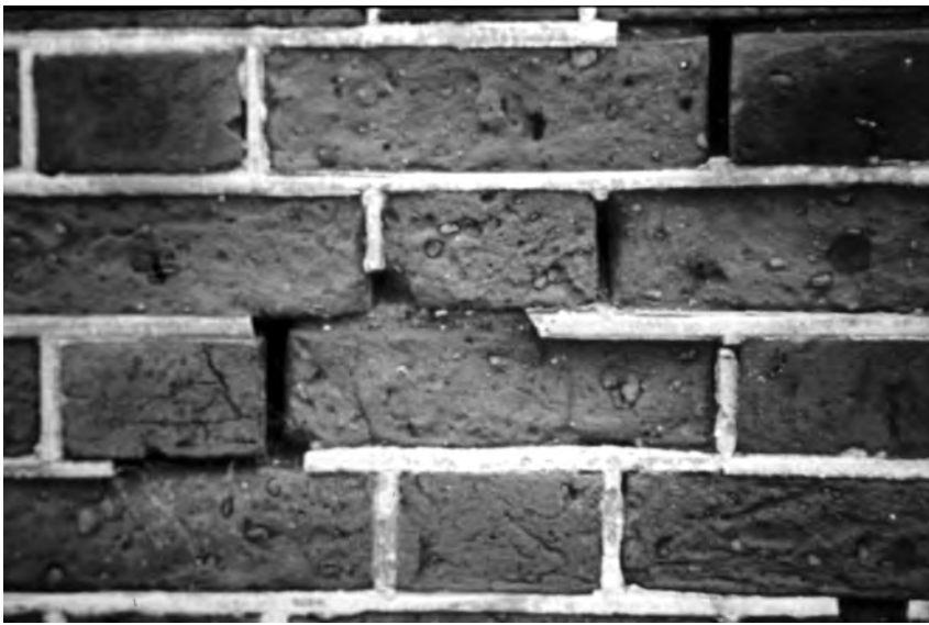
Plate 9.5 Frost damage can be exacerbated by hard cement pointing, which traps water that would otherwise drain into mortar joints and evaporate outwards harmlessly. The delay provides more opportunity for the water to freeze and split away the faces of the bricks.
