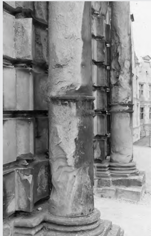
Figure 9.13 Contour scaling of sandstone caused by atmospheric pollution and cycles of wetting and drying.
