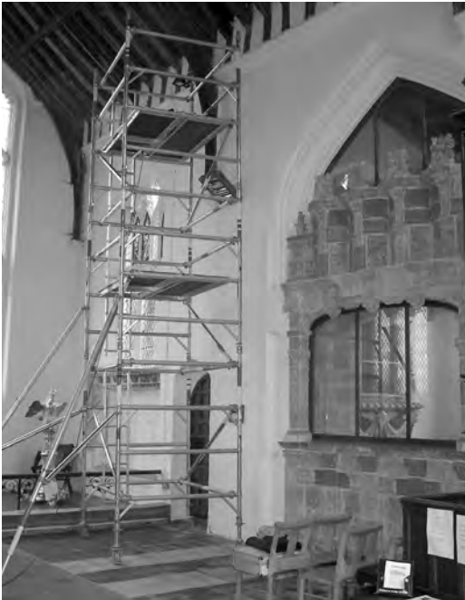
Figure 5.1a Scaffold tower used for inspection of church roof structure. Safety considerations include use of fully extended outriggers, locked wheel castors, fixed internal access ladder and platform trapdoors. Protection should be provided beneath wheel castors where there is a risk of damage to floor surfaces
