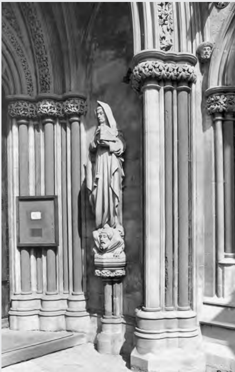
Figure 9.12 The Mansfield red dolomitic sandstone chosen by Sir George Gilbert Scott for the tall one-piece shafts to St John's College Chapel, Cambridge (1866–69) failed. The reason for this was that the stone had to be used with the bedding planes set vertically due to the shallow stratum from which the stone was taken.
