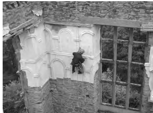
Figure 5.1d Inspection of cracking in the now floorless Great Hill Hall at Hardwick Old Hall (Derbyshire) as part of a full assessment of plasterwork condition (Credit: Joe Picalli of Conservation Solutions).
